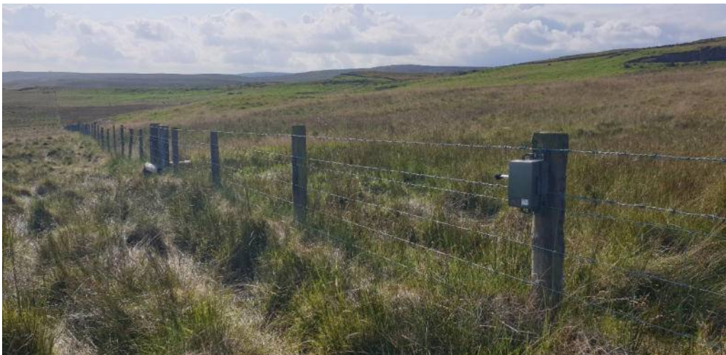
SM4 ZC with SMM-U1 microphone close to turbine Location.
