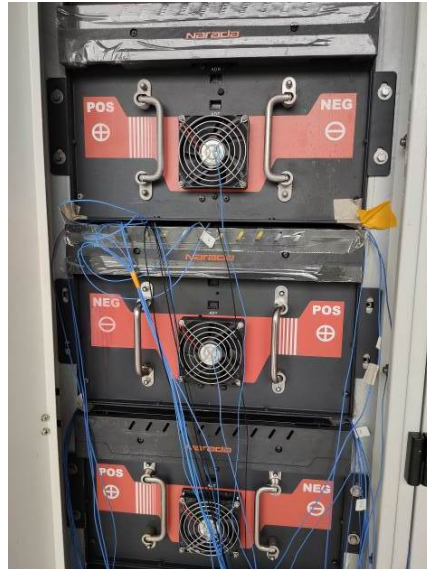
Overview – Unit after test
